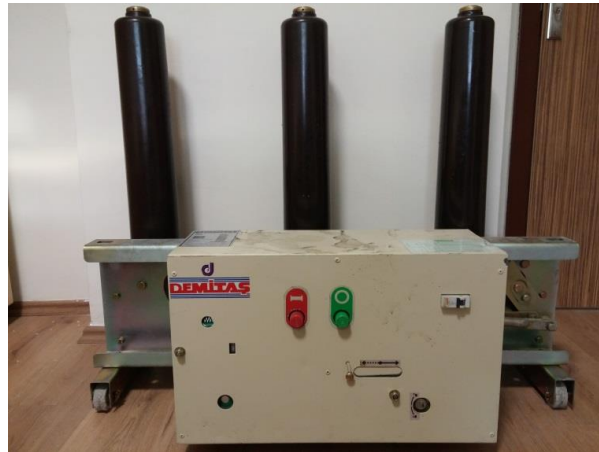
Figure 2. SF6 circuit breaker used in the project
